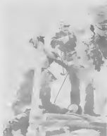
Furmanite technicians here inject a special sealing compound into holes previously drilled and tapped at # 2 Powerhouse.
